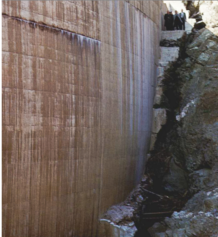
Figure 15. A large gap (crevice) displayed after the accident between the upstream face and the right abutment of the dam. Photo taken in May 1960. Courtesy of Pierre Duffaut.
