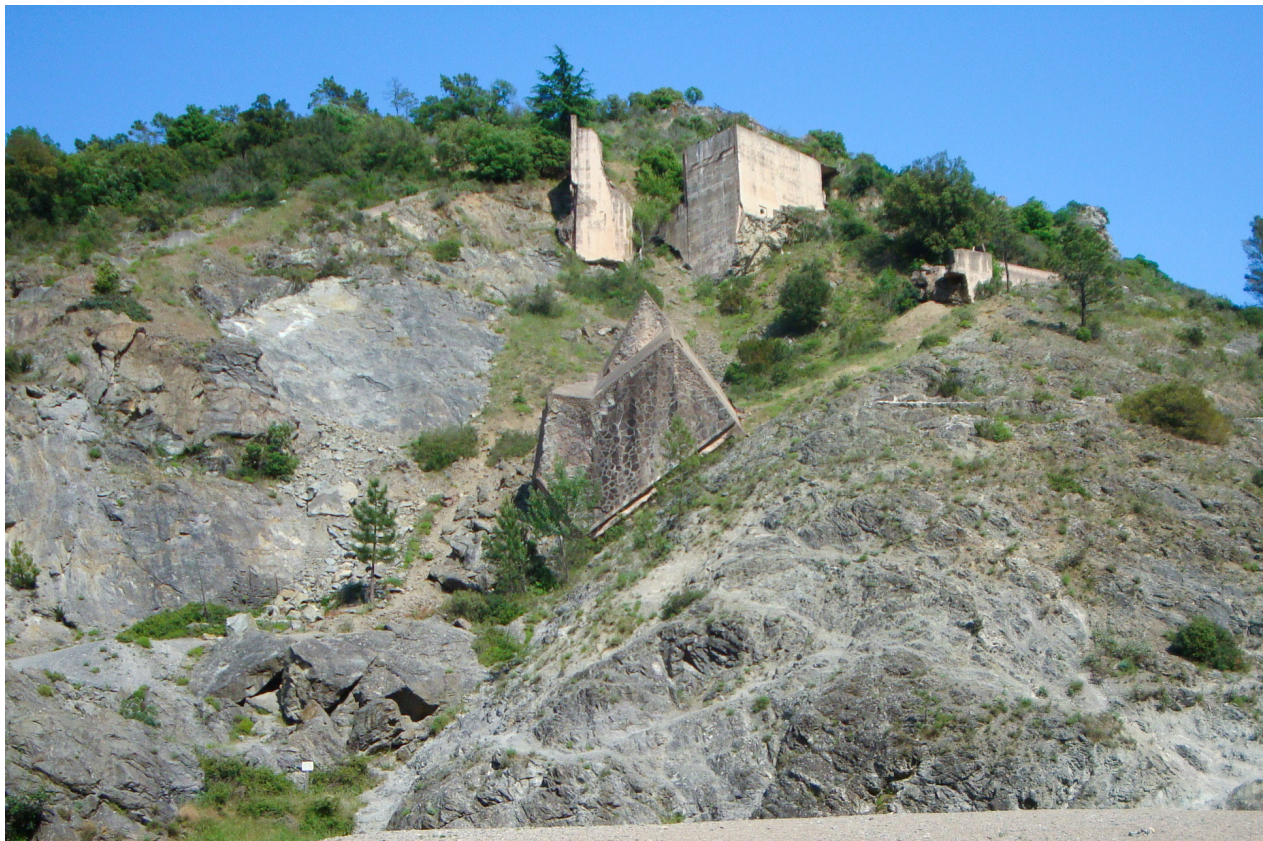
Figure 14. Damaged dam structure after the accident. Courtesy of Pierre Duffaut; Photo taken in 2010.
