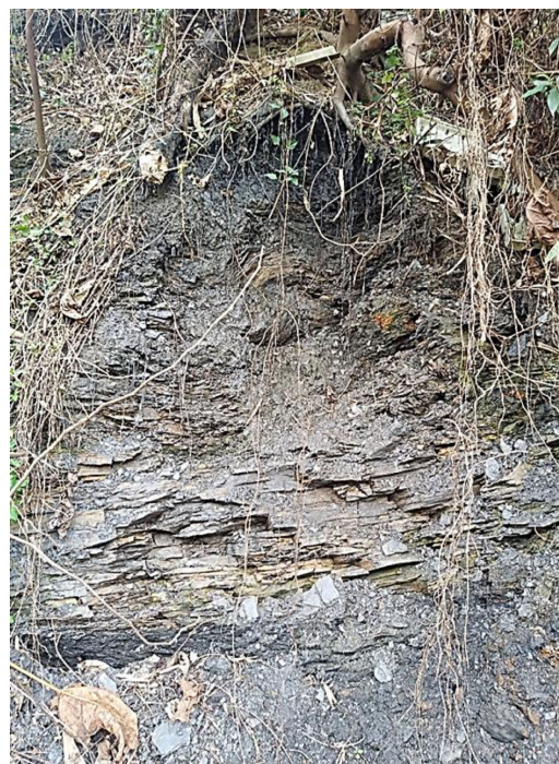
Figure 4. Bedrock at the stream bank just beneath the reported failure.
