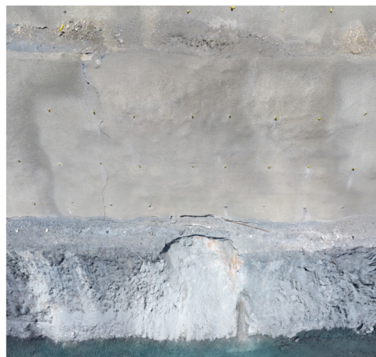
Figure 3. Visual inspection of a high-risk area using a drone (image extracted from a textured 3D model generated from drone-captured images).
