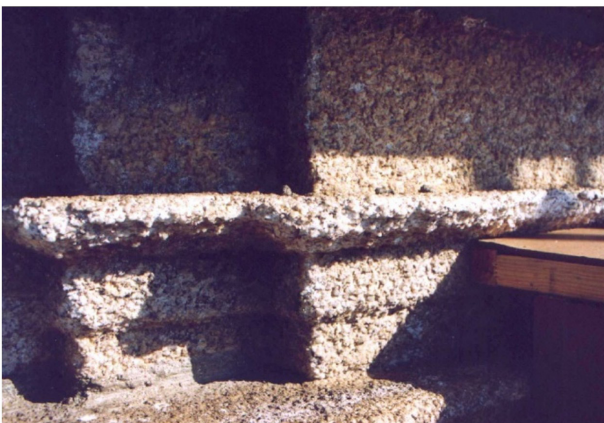
Figure 13. Disintegration of a granite block (Delgado Rodrigues, 2007).
