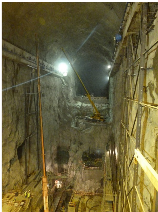
Figure 7. Frades II underground powerhouse (Lamas, 2023).
