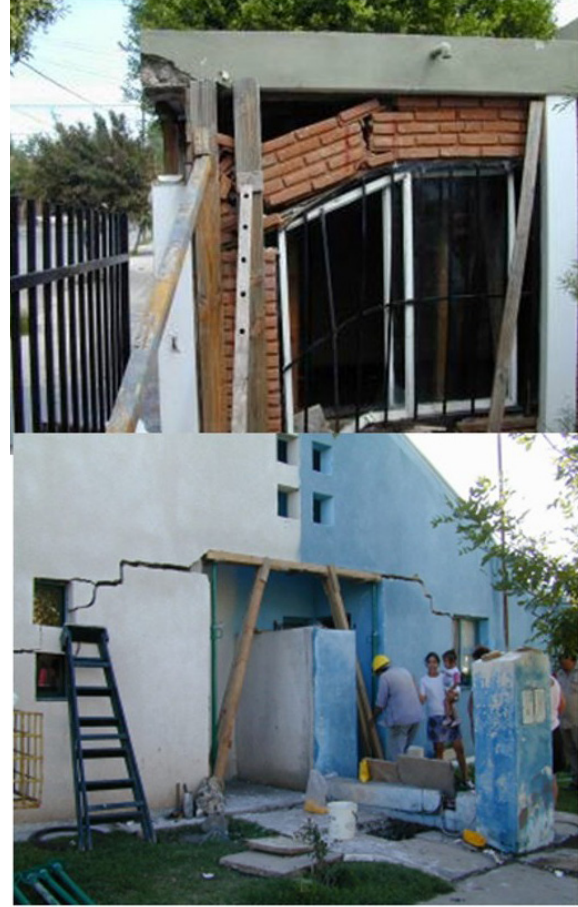
Figure 10. Damages in buildings (Terzariol, 2012).
