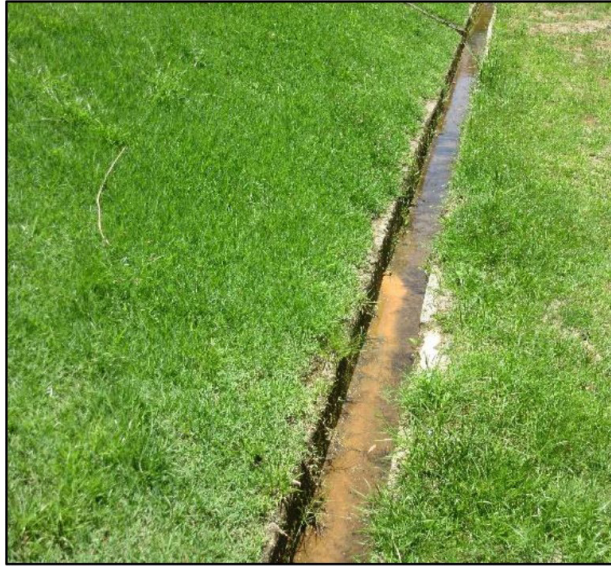
Figure 4. Evidence of fine particles being carried away in the drainage system installed at the downstream slope toe of the dam (photo taken in 2018).
