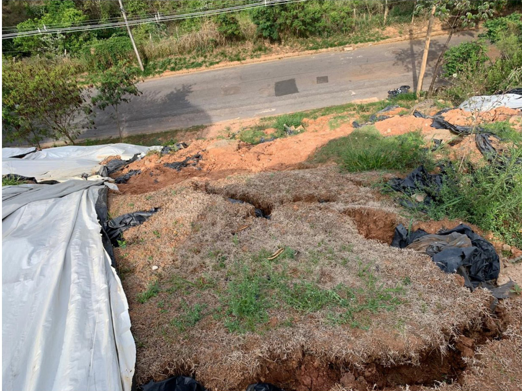
Figure 6. Erosion gullies identification alongside the slope surface.
