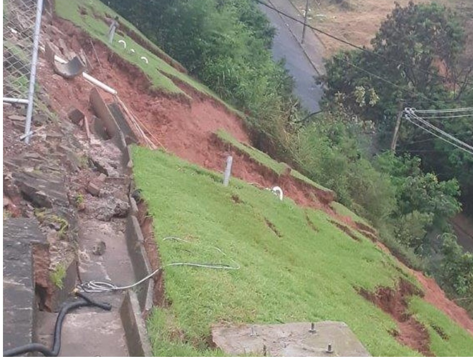
Figure 2. Soil Cracks in the surface indicating the initiation of mass movement.
