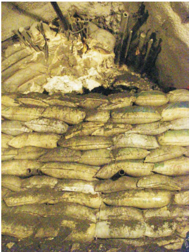
Figure 9 - Wall of injection built at Sta. 5+237.40 m, in the Pinalito rock Tunnel. Note in the roof area, part of tubes/spilling bars previously drilled and remnants of polyurethane foam.
