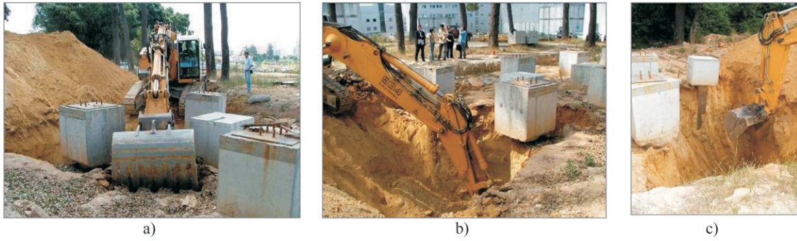
Figure 19 - Excavation: a) beginning of job; b) c) steps for soil removal (Costa Esteves, 2005).
