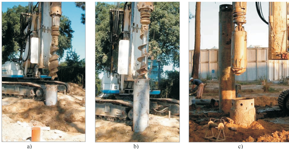
Figure 9 - Cleaning of the tube: a) and b) Borehole; c) Cleaning device (Costa Esteves, 2005).
