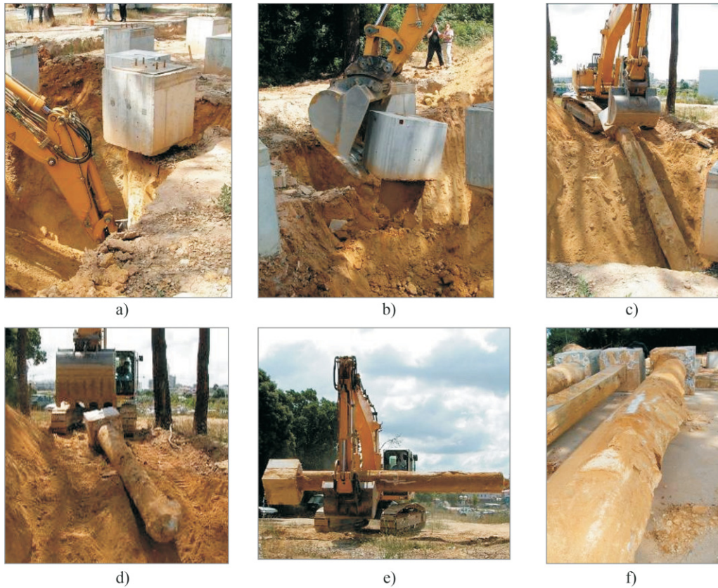
Figure 20 - Pile extraction (6 m): a) beginning of excavation; b) and c) and d) removal of pile from the soil; e) transportation of pile to the warehouse; f) general view of the pile after removal (Costa Esteves, 2005).
