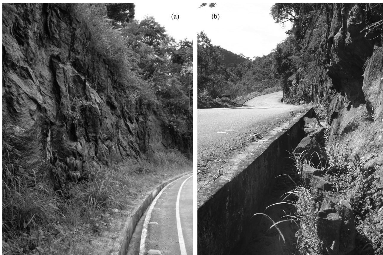
Figure 5 - (a) ES-146 slope. Presence of water is constant even in dry periods. (b) ES-355 slope. Several blocks in the ditch indicates regular rockfall problems.
