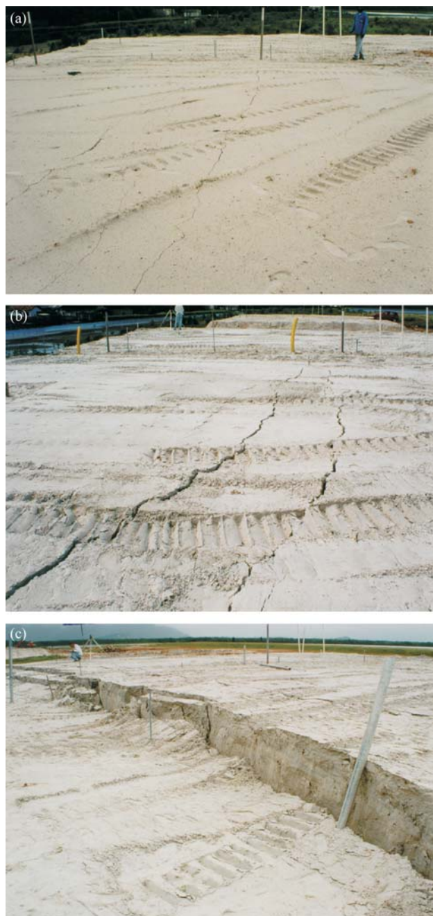
Figure 14 - Photos of the crest of the test embankments at failure.
