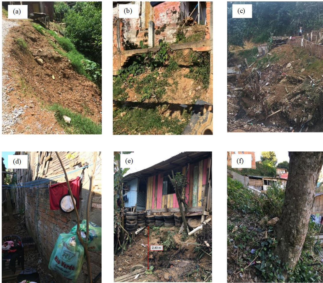
Figure 4. (a) very high susceptibility (S4): translational landslide scar of approximately 1 m depth in landfill soil; (b) very high susceptibility (S4): translational landslide scar approximately 1 m depth in landfill soil; (c) high susceptibility (S3): steps on the ground; (d) high susceptibility (S3): retaining wall cracked and bowed; (e) high susceptibility (S3): subsidence and damping by sewage deposition; (f) high susceptibility (S3): tree tilted downhill.
